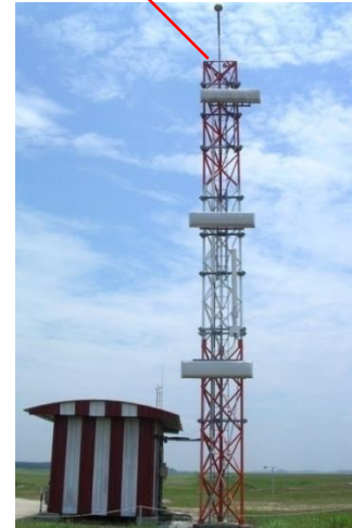
Ground Glide Path Antenna
