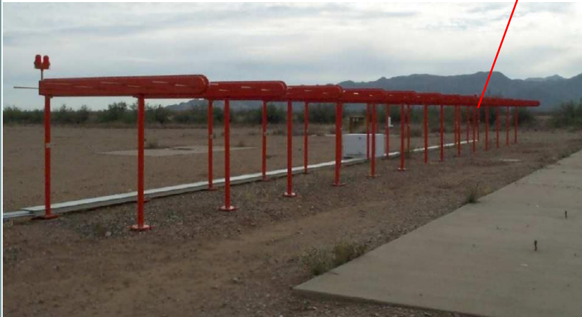
Ground Localizer Antenna
